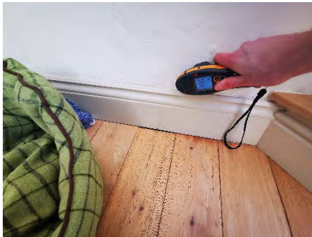
View of moisture reading.
