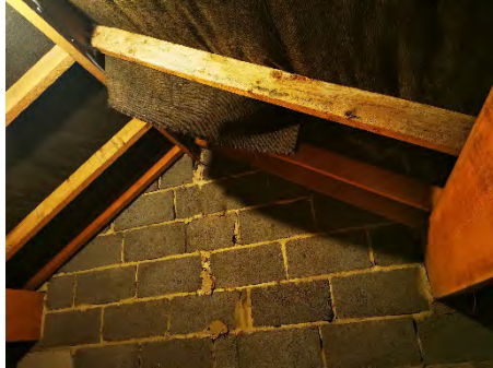
View of loose section of underlay.
