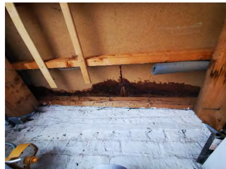
View of staining to flat roof deck.
