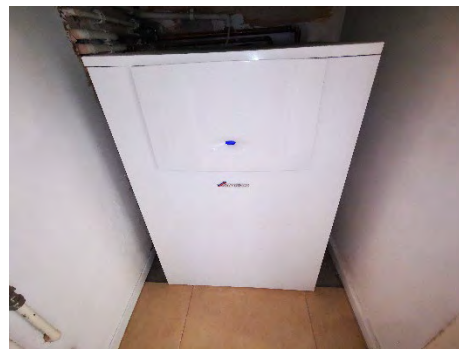
View of boiler.
