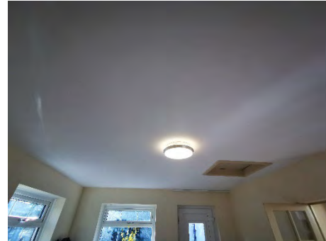
View of utility room.
