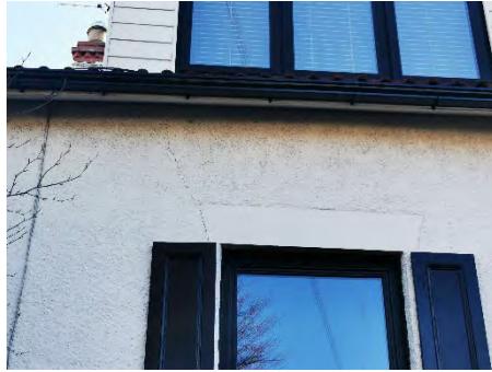
View of cracking to front elevation.
