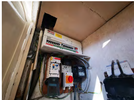
View of electrical supply location.
