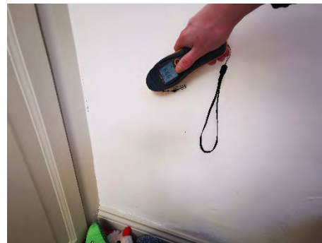
View of moisture reading.
