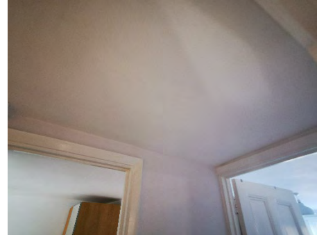
View of hairline cracking to landing ceiling.
