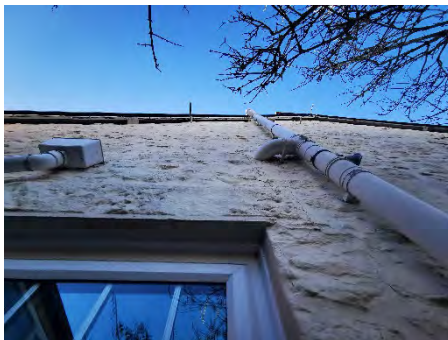
View of cracking to side elevation wall.
