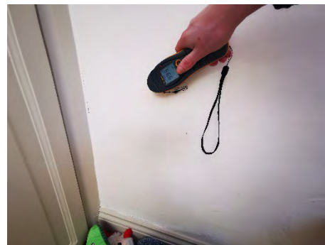
View of moisture reading.
