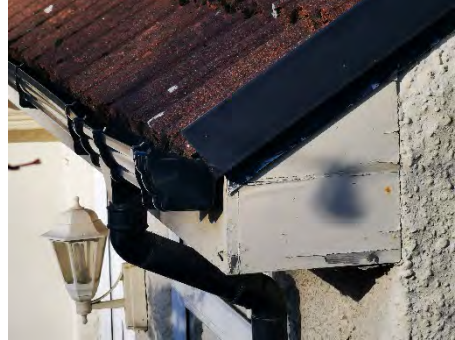
View of fatigued decoration to fascia and soffit.
