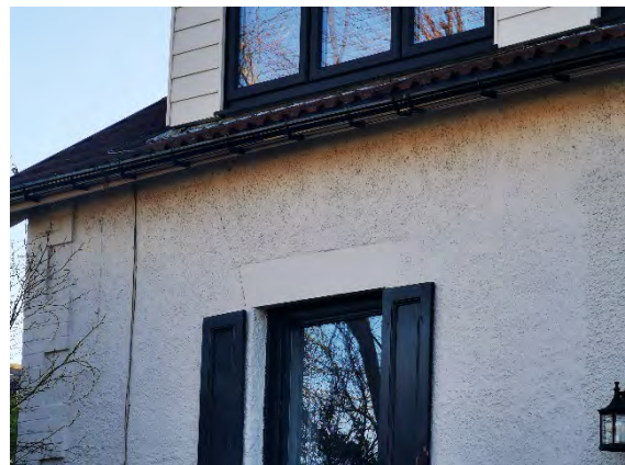
4. Cracking above window.
