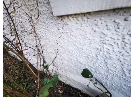
View of cracking to front elevation.
