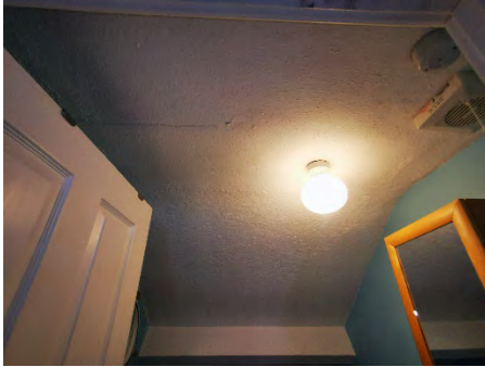
View of hairline cracking to first floor toilet.
