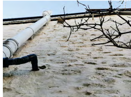
View of cracking to side elevation wall.
