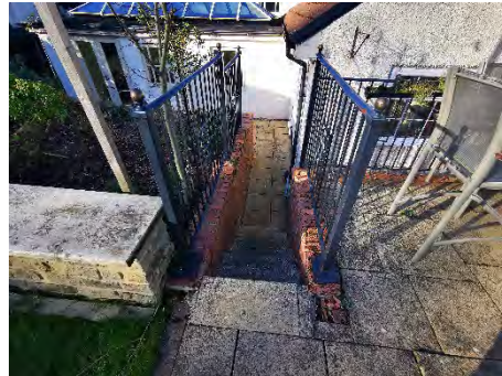
View of fatigued decoration to rear patio balustrade.
