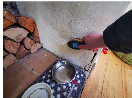
View of moisture meter reading to rear dining room fireplace.
