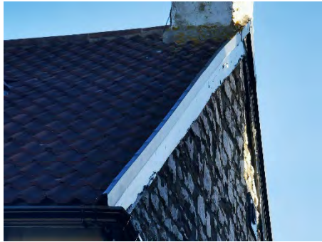
View of fatigued decoration to barge board.
