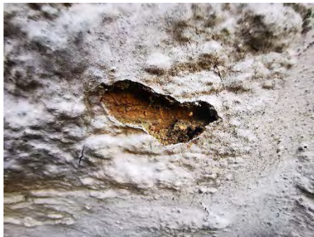
View of isolated spalling to cementitious render.
