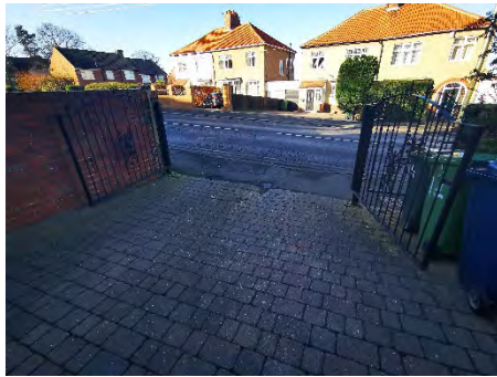
View of fatigued decoration to gate.
