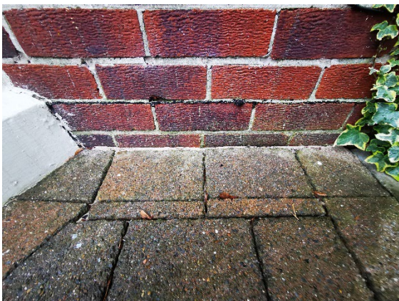
5. Suspected DPC to front elevation.
