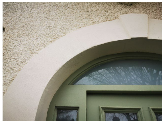
4. Hairline cracking to render finish.
