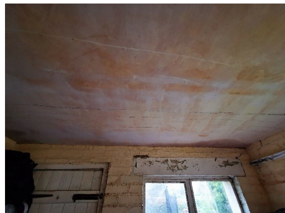
18. View of cracking to garage roof. Note cracking to external walls.
