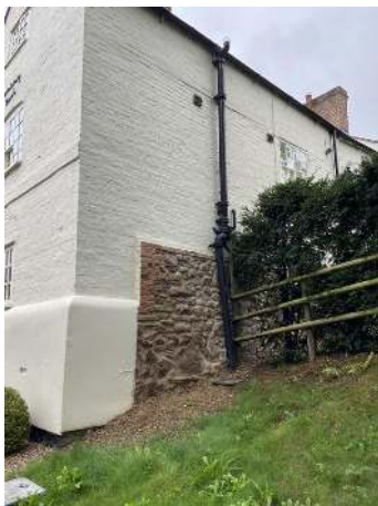
101. Soil and vent pipe
