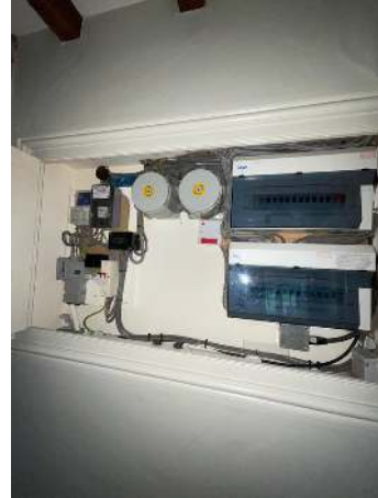
98. Electrical supply and consumer unit
