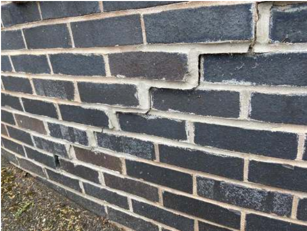
43. Boundary wall movement
