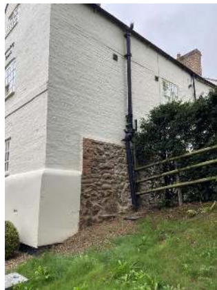
Soil and vent pipe
