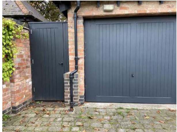
40. Driveway covering undulation noted
