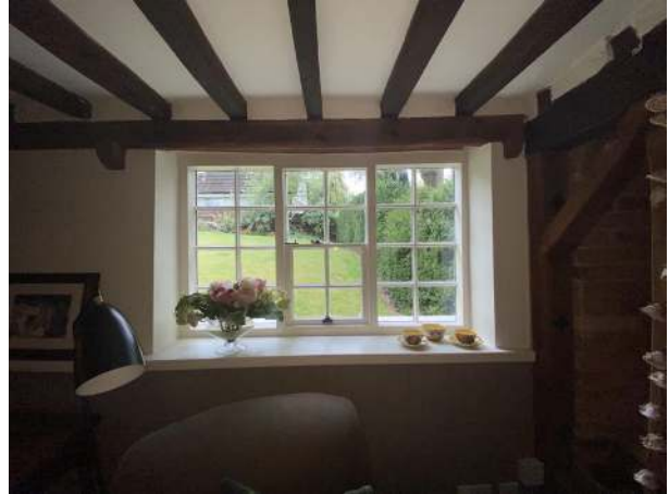
74. Ceiling affected by shrinkage
