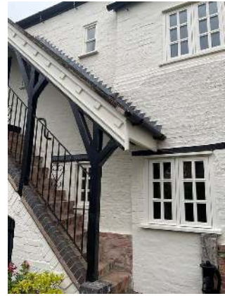
Gutter with no downpipe
