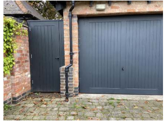
Driveway covering undulation noted
