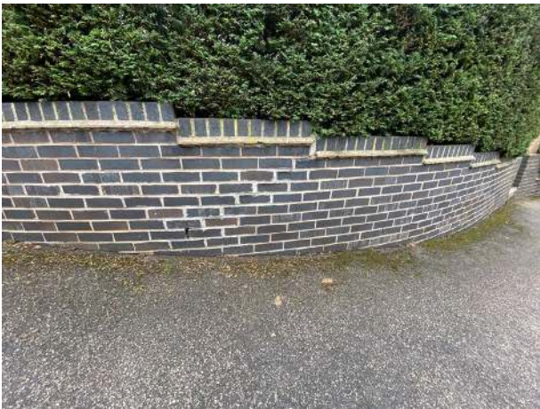
45. Boundary wall movement
