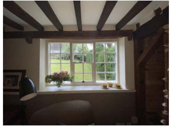
Ceiling affected by shrinkage
