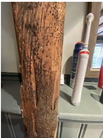
77. Evidence of wood boring beetle within first floor bathroom
