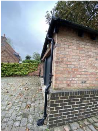
39. Driveway covering undulation noted
