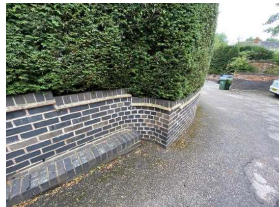
Boundary wall movement
