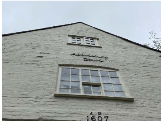
Bowing noted to side elevation
