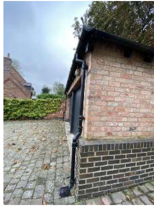
Driveway covering undulation noted
