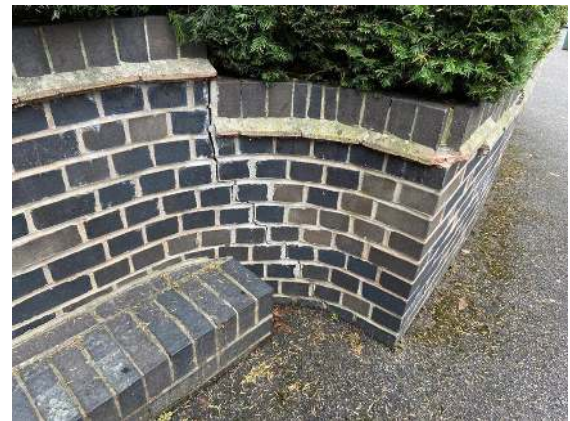
Boundary wall movement
