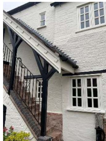
24. Gutter with no downpipe
