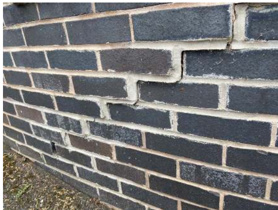
Boundary wall movement
