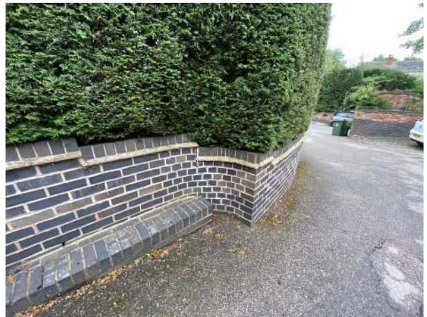
46. Boundary wall movement
