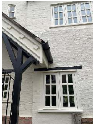
Gutter with no downpipe
