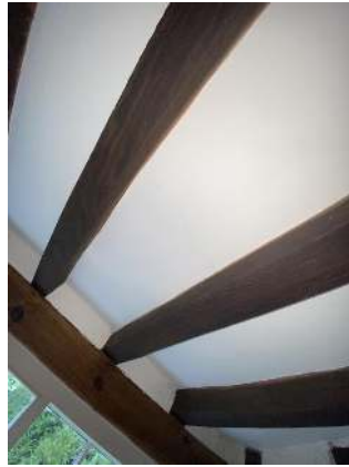
Shrinkage crack noted
