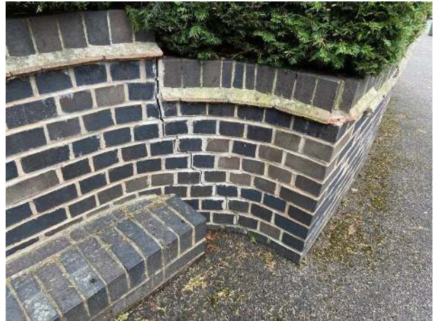
44. Boundary wall movement
