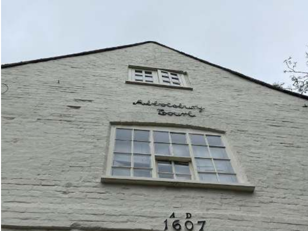
7. Bowing noted to side elevation
