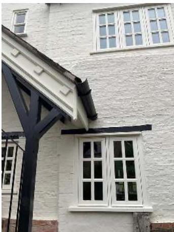
23. Gutter with no downpipe
