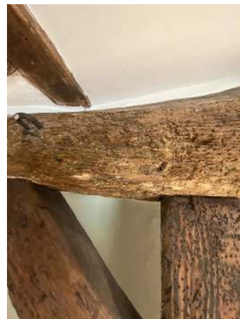
78. Evidence of wood boring beetle within first floor bathroom
