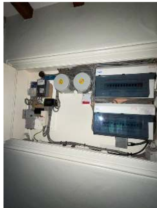
Electrical supply and consumer unit
