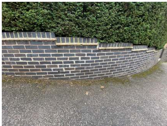
Boundary wall movement
