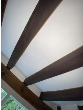
73. Shrinkage crack noted
