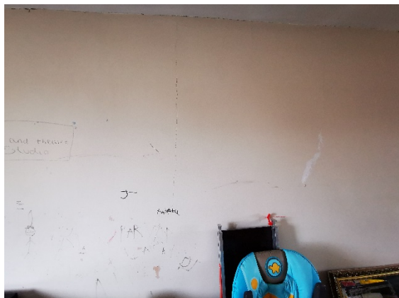
View of cracking internally to plasterwork.
