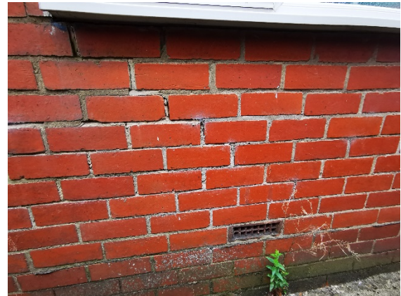
View of stepped cracking below side elevation window.
