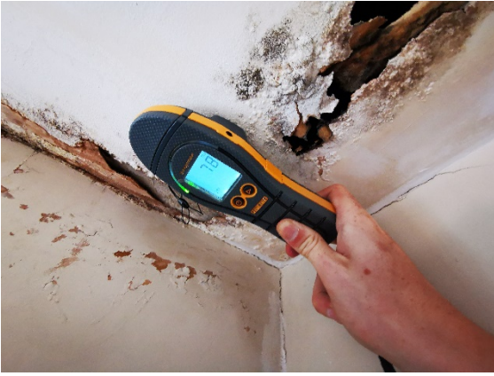
View of damage to plasterwork.
