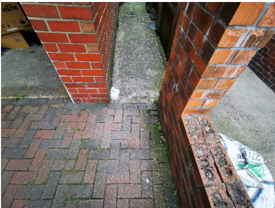
View of defected coverings to external pathway.
