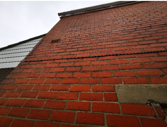
View of cracking to side elevation window.
