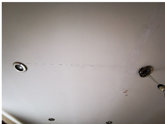
View of cracking internally to plasterwork.
